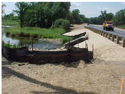
Temporary cover and silt fence work together to prevent the discharge of sediment from this construction site.
